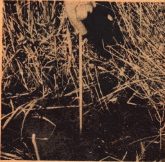
Open sewer ditch in town of Oakland. Town's 8-inch water main is less than 30 inches beneath this ditch.
